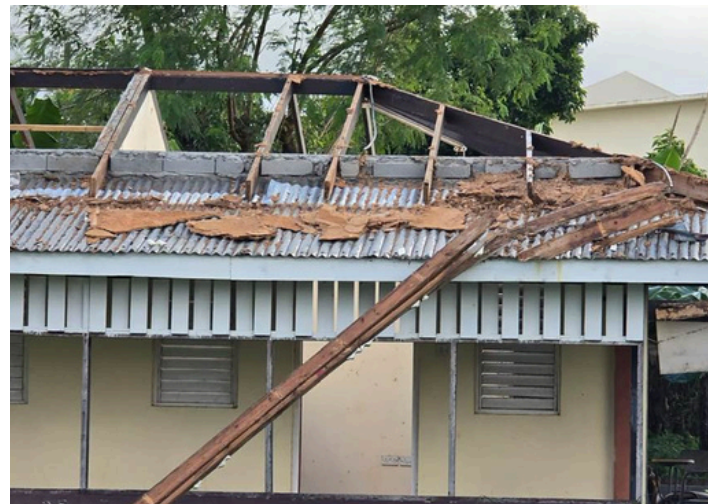
Pictured: Damage to Roof of Building on Mirabeau Campus
